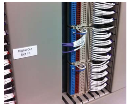
Initiator/Actuator terminals for interconnection of field devices to PLC I/O.
