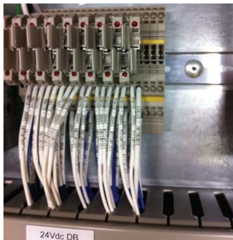
The PDL "Push In" series was used for 24Vdc distribution of digital and analogue circuits.
